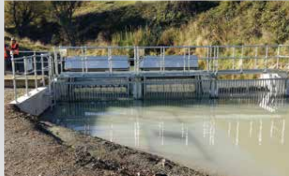
Galvanised fish screen & walkway SELWYN DISTRICT COUNCIL
